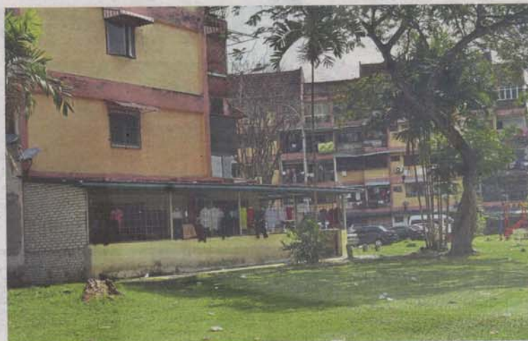
One of the ground floor units that has been extended onto the playground.
